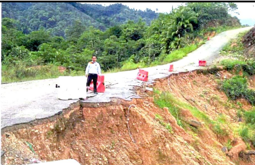
Dicing with danger: Abun visiting the site of the eroding hillslope along the Belaga-Menjawah road in northern Sarawak.
